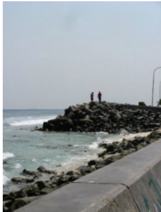
Figure 7. Tetrapod barrier along Male's western coast, bordering land created during the Male' Land Reclamation Project. The tetrapod barriers interlock, and are anchored in coral rubble (blackened by sun exposure and algae) and are backed up by a concrete barrier wall (photo by the author, April 2010).
